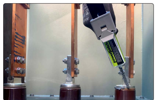
Leaking Switchgear Repair
